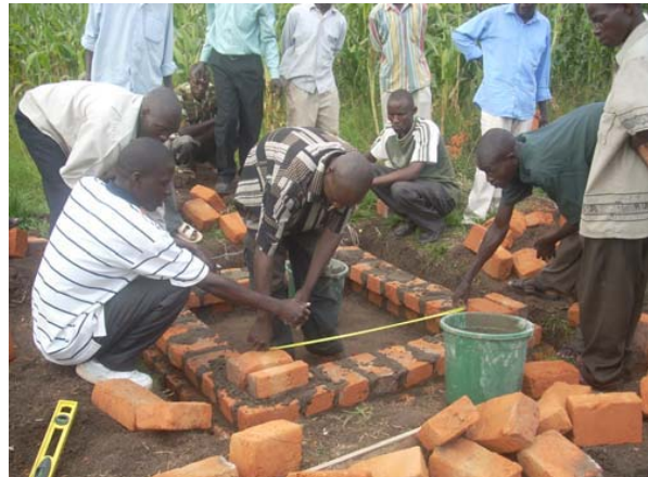
Masons undergo training in construction of improved latrines, developed by HIP's SanMark activity in Tororo District.
